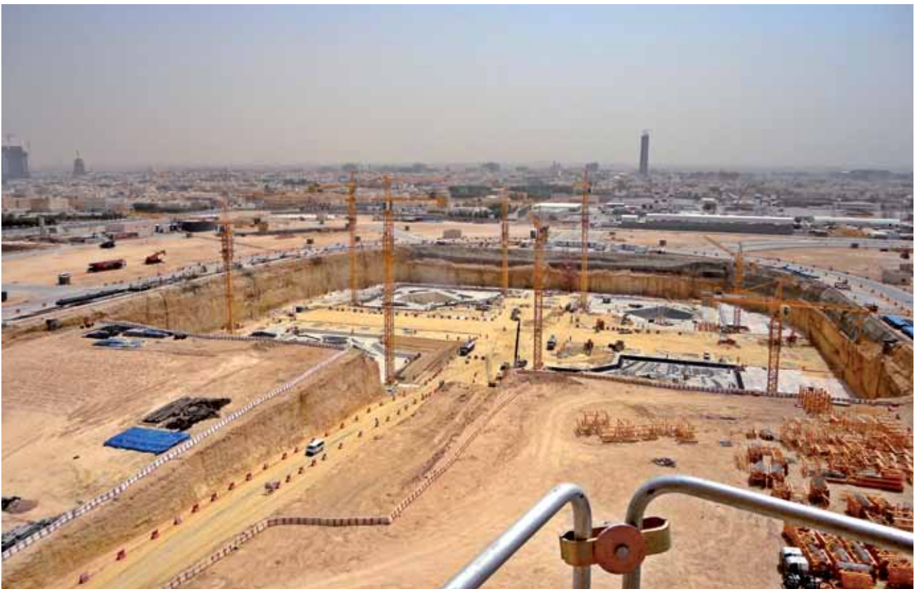
The construction site of the Information Technology and Communications Complex (ITCC) ▼ Riyadh, Saudi Arabia
